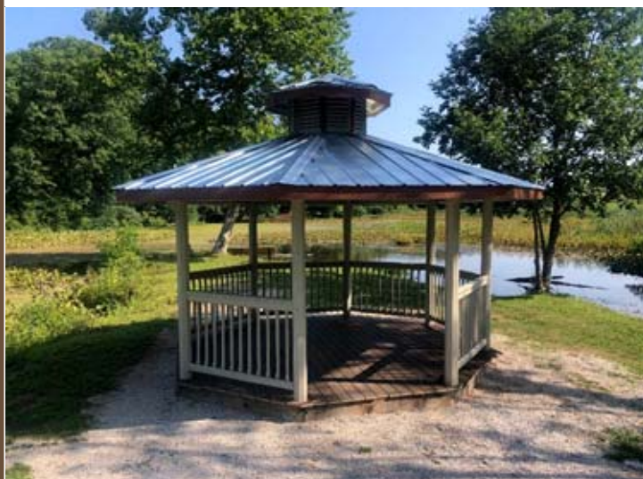
Nearly complete reconstructed gazebo in its new location at Red Mill County Park.
